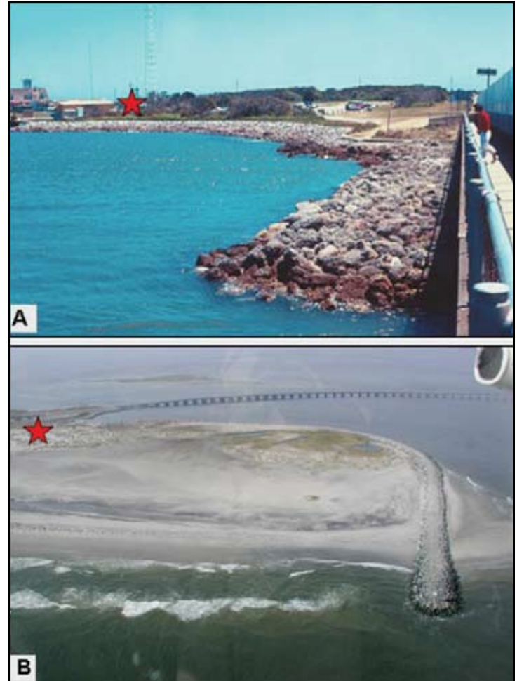
FIGURE 14. Photographs of the Oregon Inlet bridge with a rock revetment built in 1989 around the south end of the bridge to secure it to Pea Island (Panel A) and a jetty built in 1989-91 to stabilize the south shore of the migrating inlet (Panel B). The red star shows the location of the former U.S. Coast Guard Station. Photographs are by S. Riggs.
