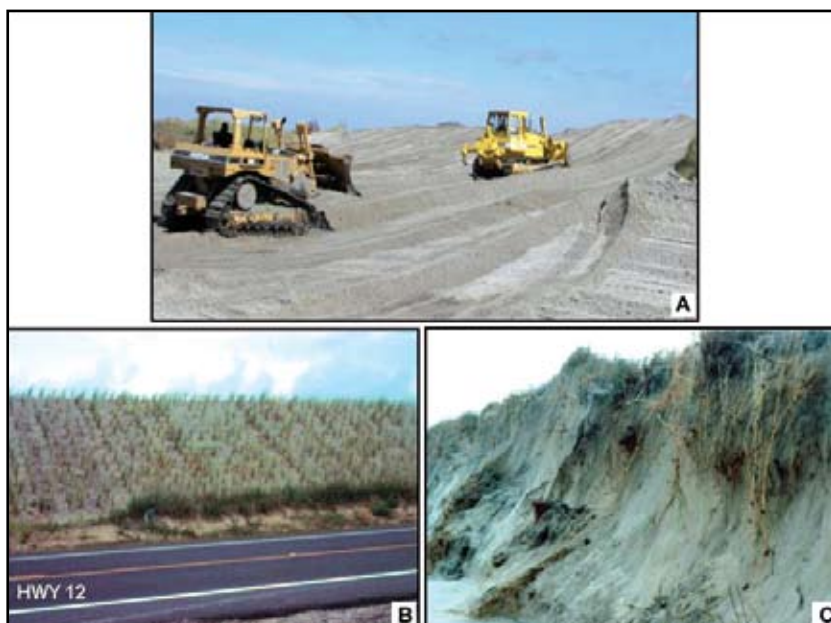
FIGURE 16. Barrier-dune ridges are constructed today with NC DOT bulldozers (Panel A). The dunes are fertilized and grassed (Panel B) in an effort to protect NC Highway 12. Because the barrier-dune ridge is out of equilibrium with beach dynamics during storms, the dune ridge is eroded and scarped on the ocean side (Panel C) and will, ultimately, be breached. Photographs are by S. Riggs.
