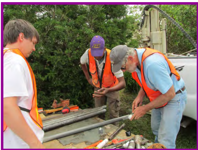
James Owers, John Woods, and Alex Manda examine sediment in a core while constructing a monitoring well on Bogue Banks.
